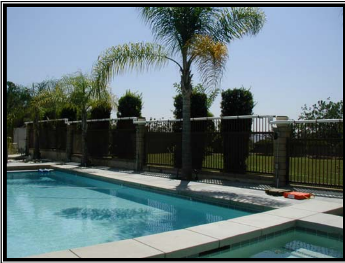
This iron fence was modified to accommodate our solar piping along the top.
